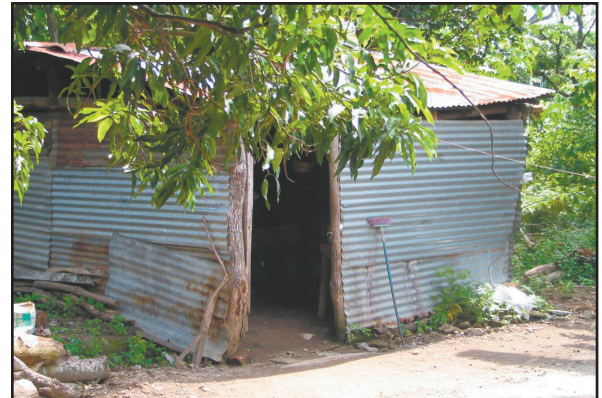
BEFORE: Many of the homes are on the verge of collapse.
